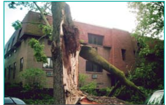
Fortunately, Sasser Family House sustained only minor roof damage when a tree fell on the building during a recent storm.
